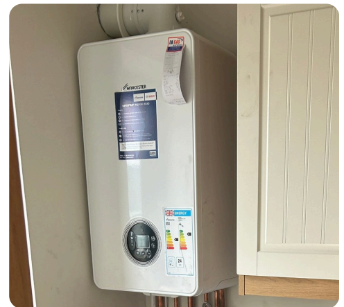
Gas Boiler Option: Combi Boiler in the Utility, with Programmable Thermostat
